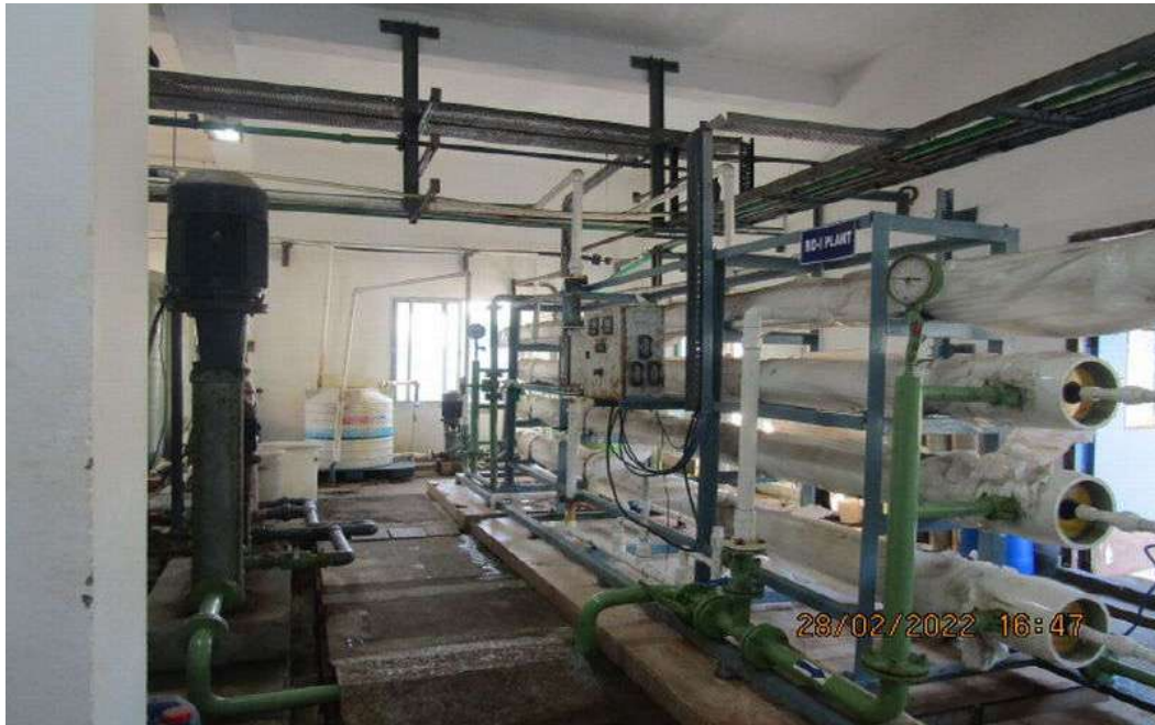
Ro System Photograph
