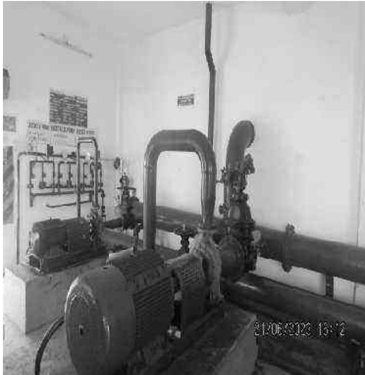
Fire fighting system Photograph
