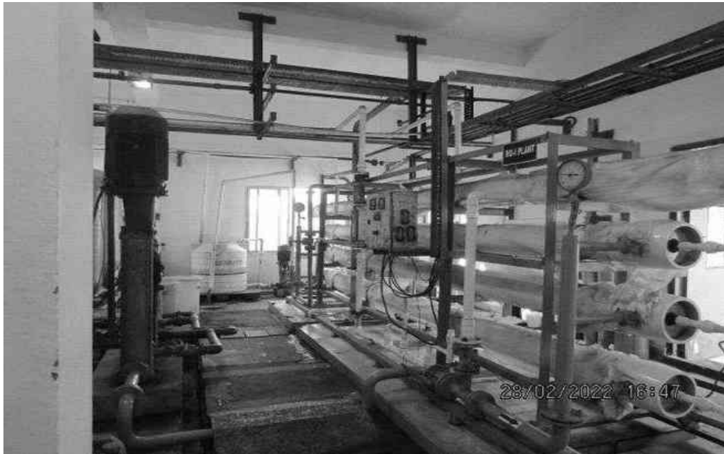
Ro System Photograph
