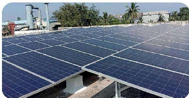
Solar Panels are installed at Roof top of Puducherry of capacity 364 kW
